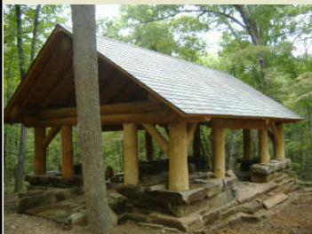
the New Pavilion is nearing completion, -Pete Hienzemann reports that only three small rocks remain to be placed in the floor.
