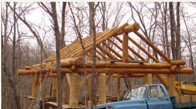
Nearing Completion, The Pavilion in Mount Sequoyah Woods Photo by Duane Woltjen
